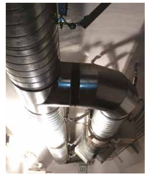
Ten mechanical rooms connect north and south bound tunnels.
