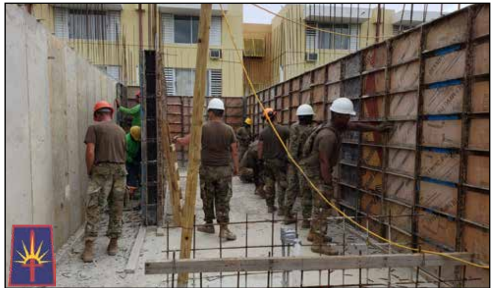
Soldiers of the 204th Engineer Battalion at work on the construction of a three-family home being built by Habitat for Humanity in San Juan, Puerto Rico on August 7, 2018. The battalion sent 45 Soldiers to Puerto Rico to assist in the construction as part of the Department of Defense Innovative Readiness Training Program. Photos by Maj. Dan Colomb, 204th Engineer Battalion.
