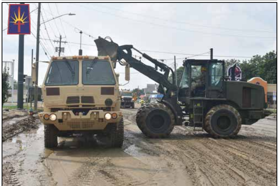
New York Army National Guard Soldiers assigned to the 827th Engineer Company respond to flooding in Binghamton, N.Y., Aug. 15, 2018. Soldiers were responding to flooding throughout many areas of Binghamton assisting civilians and the Department of Transportation. Photo by Spc. Andrew Valenza, Joint Force Headquarters.
