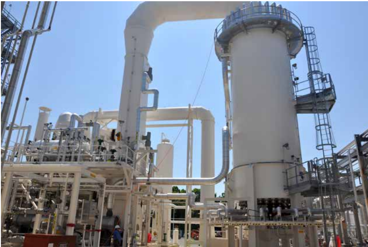
Pan American Hydrogen built the components of this Mississippi hydrogen generating plant in the Rio Grande Valley and installed it on site. Footprint of the plant is approximately 60 feet by 90 feet. (Courtesy)
