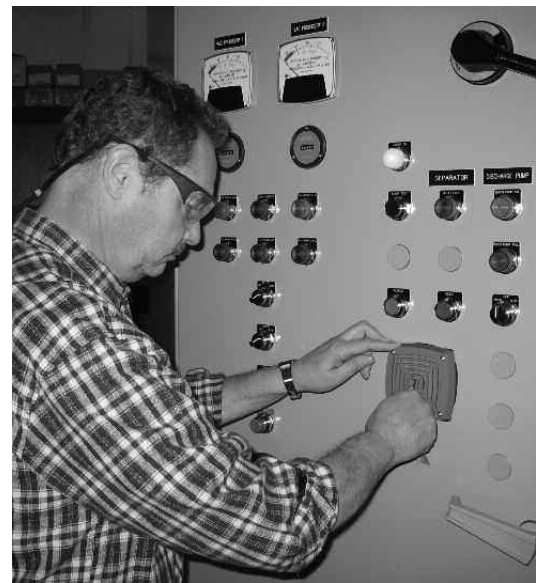
Simple to complex control panels are designed and built by Spencer's Electrical Controls Engineering and Manufacturing departments.
