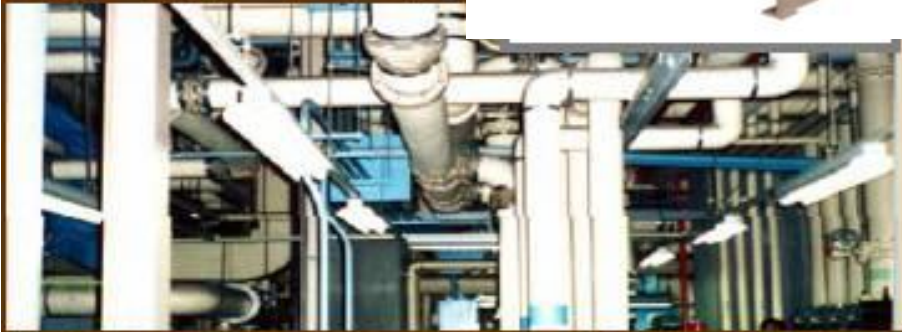
PIPING above CHILLER
