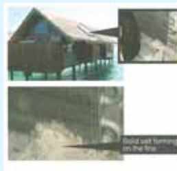
Rooftop with Strong Sea Breeze Strong sea breeze blowing directly to coil can shorten the life of the coil.
