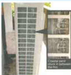
Sandy Location Coastal sand stuck in between the fins causes damage to the protection coating.
