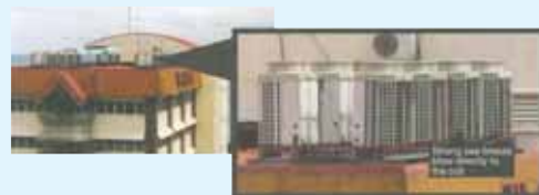
Enclosed Area and Sea Water Splashing Condition Sea water splashing directly to the coil causes solid salt forming on the fins coating.
