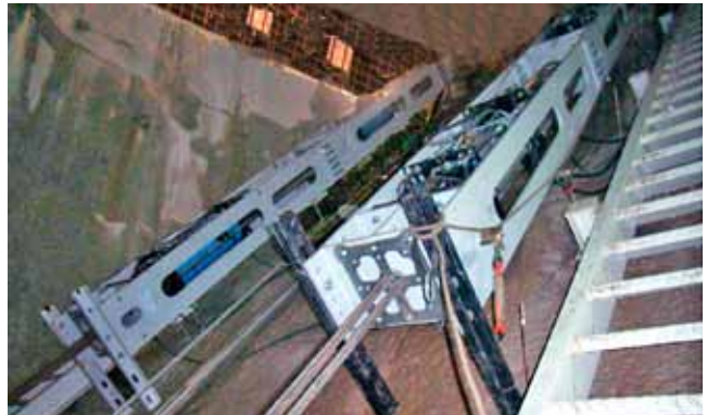
For the lifting and lowering operations at Europe's largest pumped storage plant, VSL Heavy Lifting developed a new tandem lifting/lowering system that allowed speeds of up to 40 m/h to be achieved. La Muela Hydroelectric Power Station - Spain (2009-2010)
