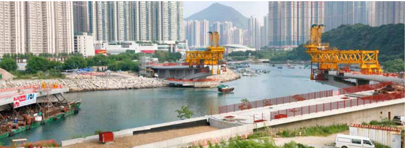
A 1,600 t centre span with a length of 55 m was lifted into place. Tseung Kwan O Bridge, Hong Kong - China (2012)
