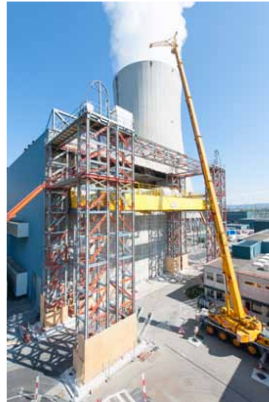
A machine-house gantry crane was replaced with a larger one. Power Plant, Gösigen - Switzerland (2012)
