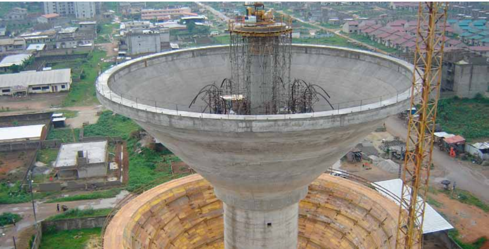
A 2,700t storage tank was lifted by 35 m. Abidjan Water Tower - Ivory Coast (2008)
