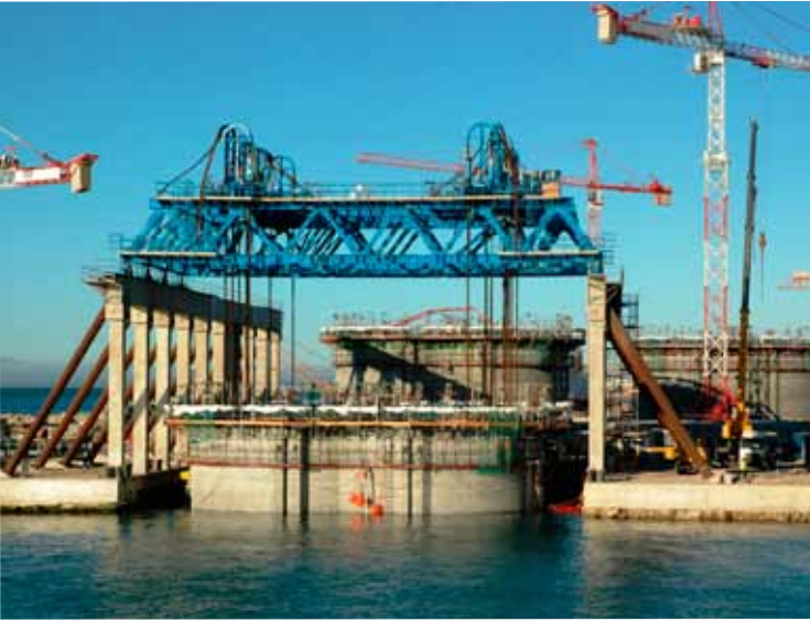
More than 100 caissons were skidded and then towed into position to create new breakwaters. Tangiers Med 2 container port - Morocco (2011-2013)
