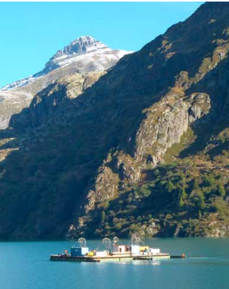
Two 2,000t concrete caissons were lowered about 100 m onto the ground of a reservoir. Dam Reservoir, Emosson - Switzerland (2011 and 2012)
