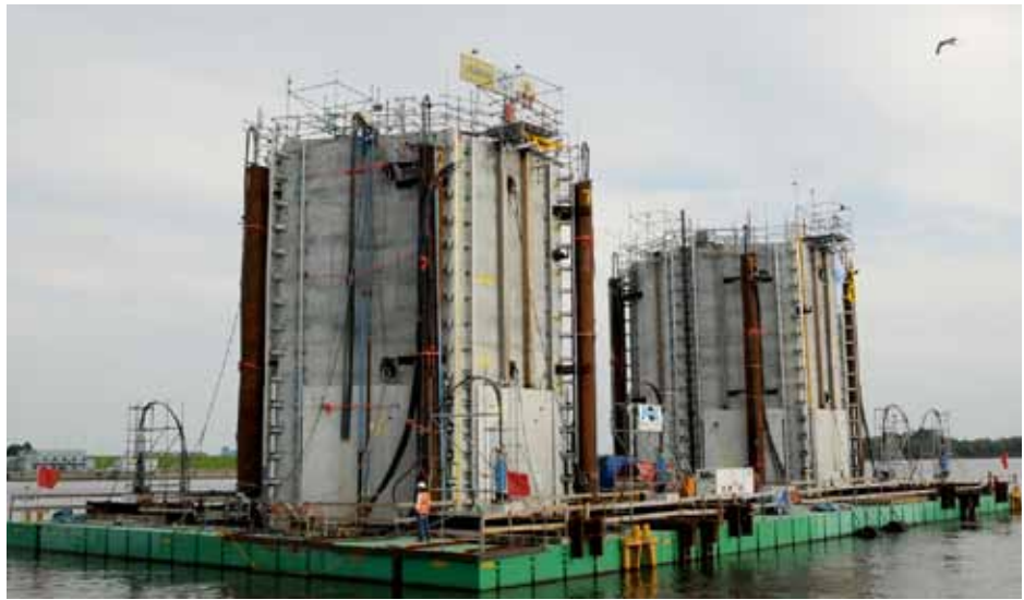
Cooling towers for a power plant were built in a dry dock before being transported by sea and then lowered into the water onto their foundations. Electrabel Power Plant, Wilhelmshaven - Germany (2013)
