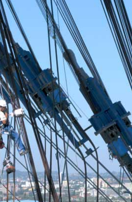
The new stadium in Durban has a remarkable roof structure: a giant Y-shaped arch representing the South African flag. Its construction required the special installation of 'flying' - or self-climbing - strand jacking units. Moses Mabhida Stadium, Durban - South Africa (2008-2009)
