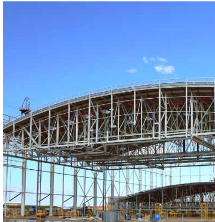
The roof of a massive aircraft hangar was lifted in two parts, weighing 970 t and 770 t. A380 Hangar, Toulouse - France (2013)
