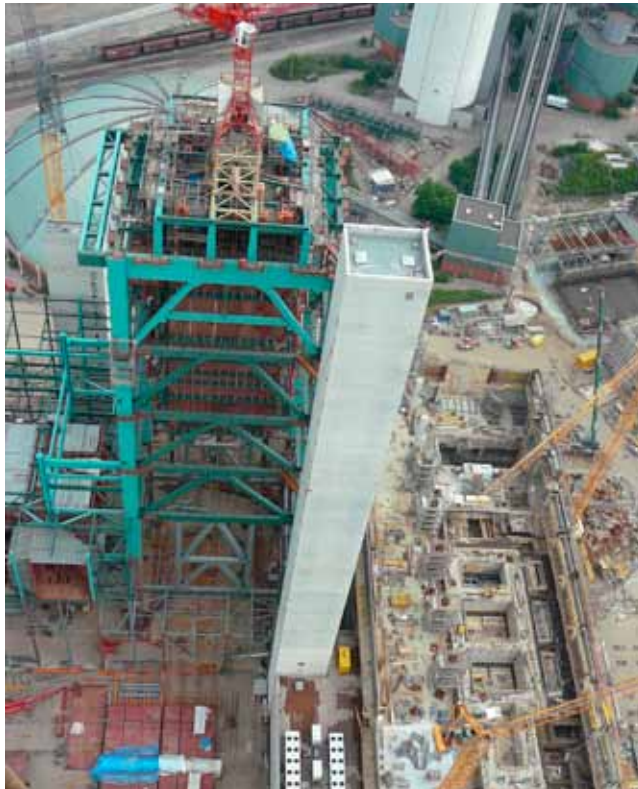
VSL lifted a power plant's steel boiler components and some of the pipework. Power Plant Walsum Block 10 - Germany (2007-2008)
