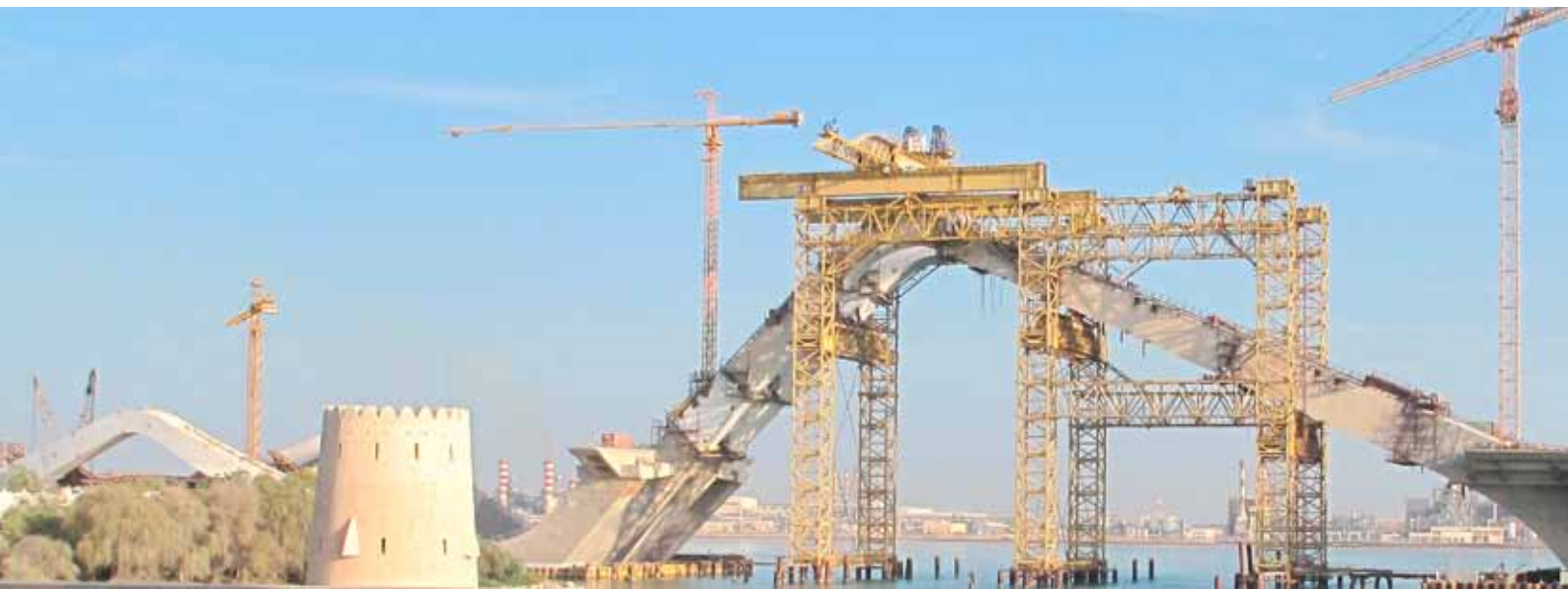
Erection of arch segments for a striking 843 m-long bridge wouldn't have been possible without the expertise of the VSL Heavy Lifting team. The bridge's curved design symbolises sand dunes in the desert. Sheik Zayed Bridge, Abu Dhabi - UAE (2006-2010)
