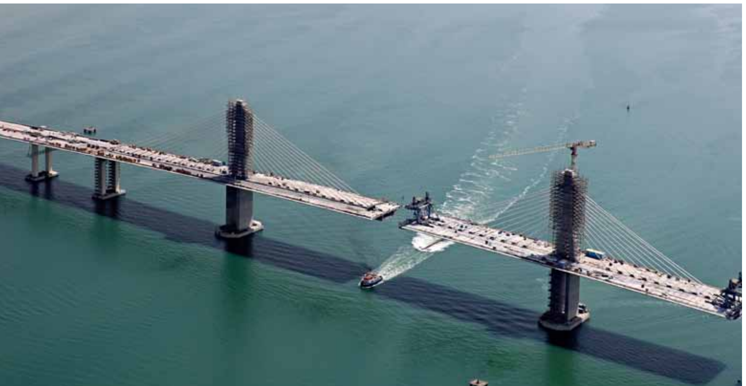
VSL designed and built a 1.3km-long six-lane cable-stayed bridge, connecting the western coastline of Abu Dhabi with Hodariyat Island. Hodariyat Bridge, Abu Dhabi - UAE (2009-2012)
