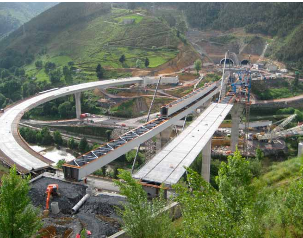
Space restrictions led to the development of a totally new method for launching the steel structures of two main viaducts. Cadagua Viaduct, Bilbao - Spain (2009 - 2010)
