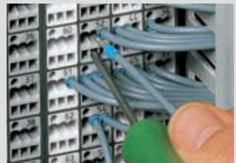
Connection of ferruled wires
