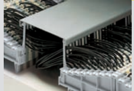
When using terminal blocks with locking strips the wiring space between the terminal strips can be covered with a wiring duct cover*. (*for suitable suppliers – please contact factory)
