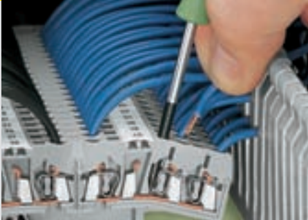
Terminal blocks for matrix patching. Connection/removal of wires on the terminal blocks sides
