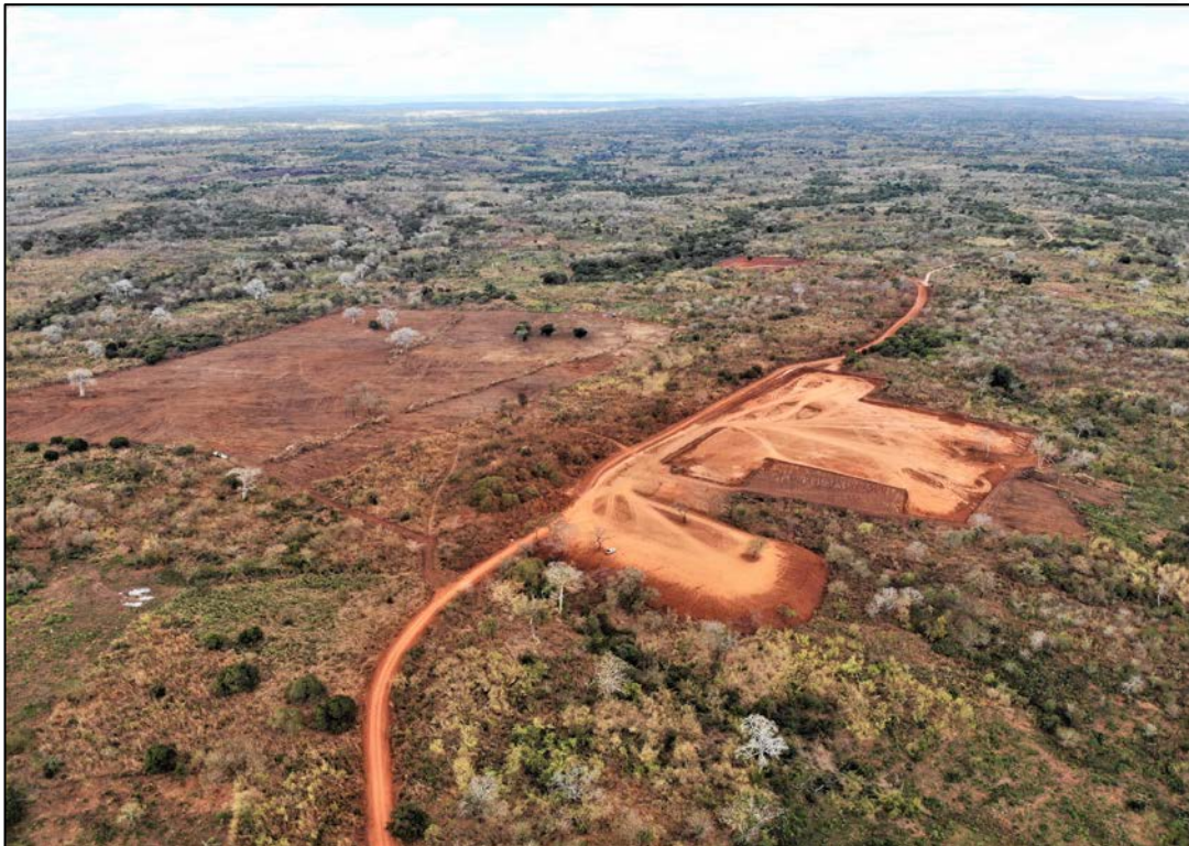
Figure 3: Aerial view from the southwest of the earthworks completed including the ROM and Processing Plant area in the foreground and clearing for the TSF area directly towards the north.
