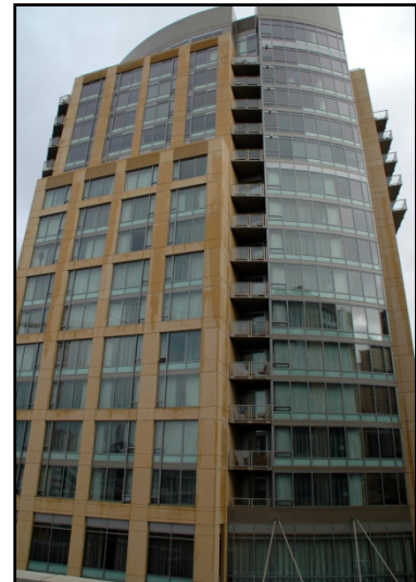
Saturated Precast Panels
