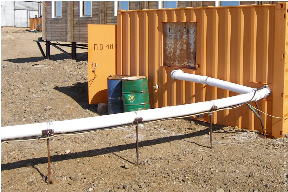
Figure 4 – Heated wastewater pipeline at Progress station (2006)
