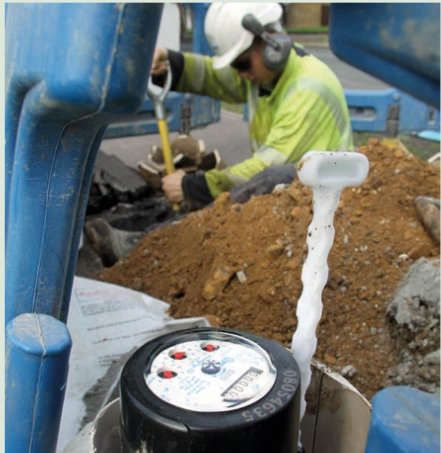
Southern Water opted for AMR meters in its major metering programme
