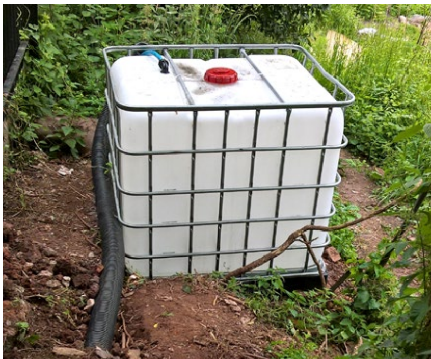
Water storage used in RainShare's pilot installation in Exeter
