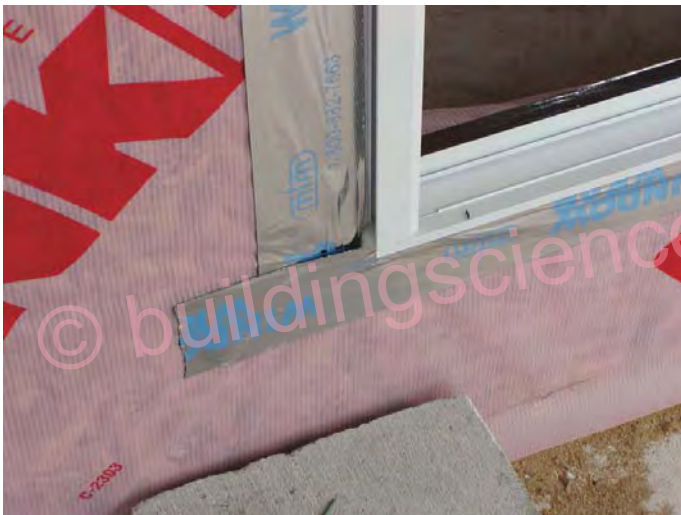
Figure 23: Reverse lap of self adhered membrane at window sill in a barrier installation
