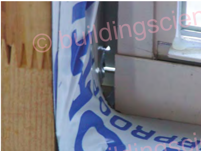
Figure 28: Window corner cutting into improperly seated pan flashing
