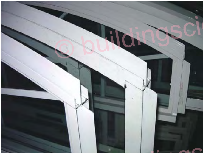
Figure 20: Discontinuity of the nailing flange at the corners
