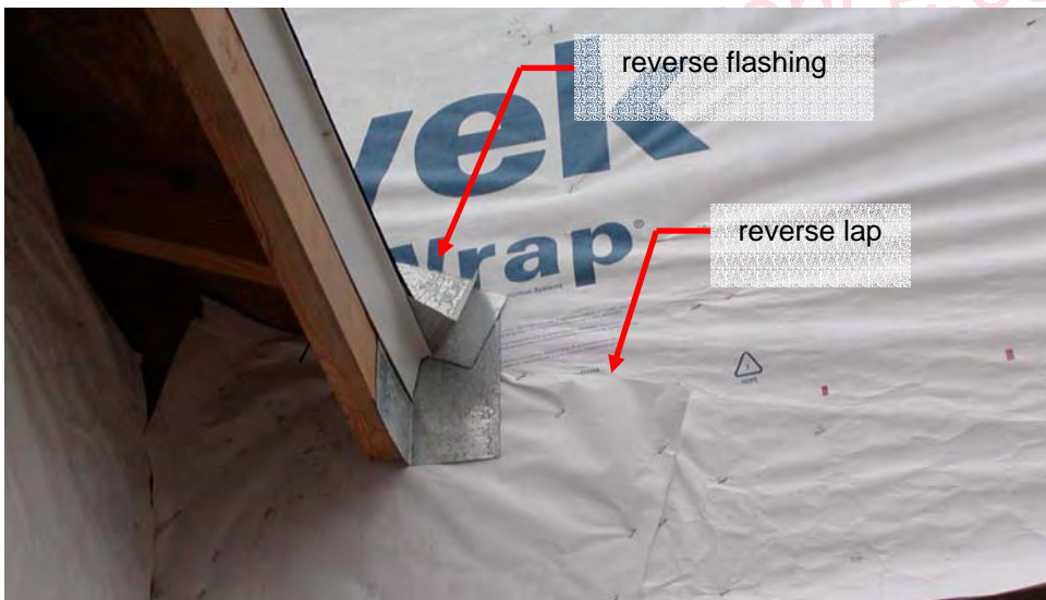
Figure 2: Improper installation of drainage plane materials
