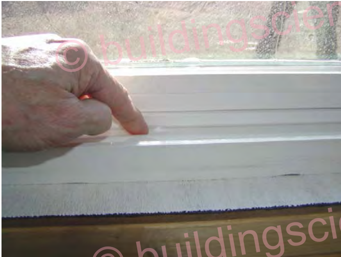
Figure 19: Water intrusion through the window frame
