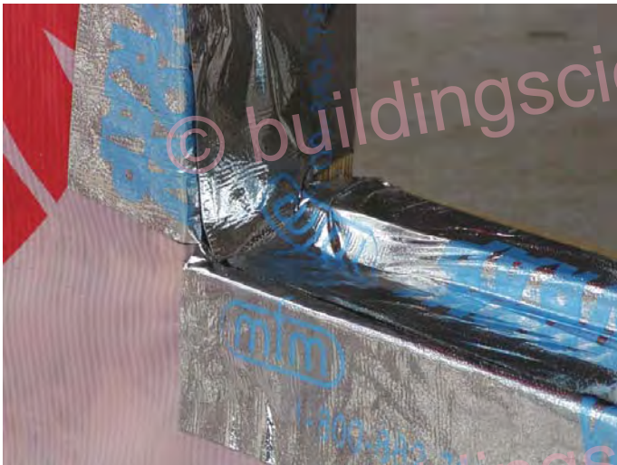
Figure 26: Tenting of the membrane pan flashing in the corner
