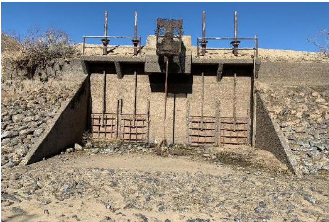
Black Canyon Main Canal Gate in off-season (2021).
