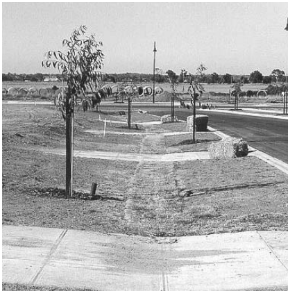
Grass cover along the swale is established using rolled turf and hydroseeding. Hay bales are placed across the kerb chutes and driveway inlet pits are sealed to protect the system from sediment laden runoff during construction.
