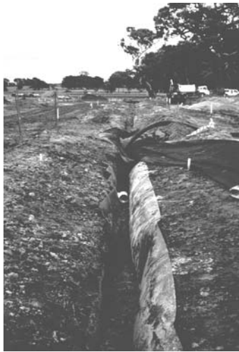
Laying of the geotextile fabric and 150mm diameter perforated pipe along the trench of the bio-filtration system. Root barriers are used where trees will be planted.
