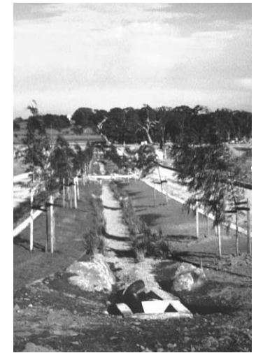
Early landscaping activities showing the gravel base of the swale that extends into the underlying trench.
