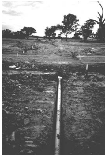
Roof runoff from the allotments located on the high side of the road drain to the gravel trench using a PVC pipe.
