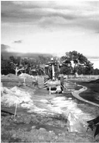
The general shape of the swale is graded using the kerb to guide the distance to the centre of the system.
