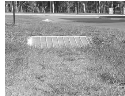
When the discharge capacity of the system is exceeded, stormwater is conveyed as open channel flow on the grassed swale to a grated entry pit at the downstream end of the system.
