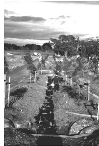
Geotextile fabric is temporarily used to protect the gravel trench from sediment in runoff during landscaping activities.
