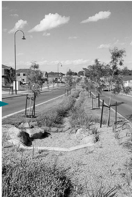
The bio-filtration system forms the median strip with the road's cross fall sloping towards it.
