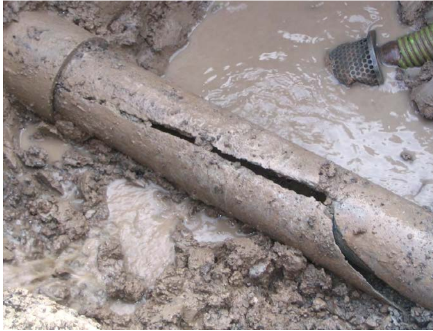
Figure D-3: Longitudinal watermain break with evident Contamination .
