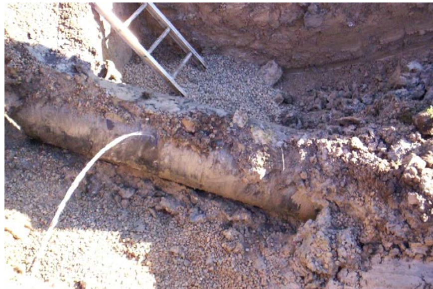
Figure D-2: Corrosion hole leak in a watermain with flow maintained until after an Air Gap was established.
