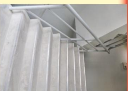
Stairs are the safest way out of a tall building during a fire.
