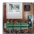
PCB, Power trans, Terminal block
