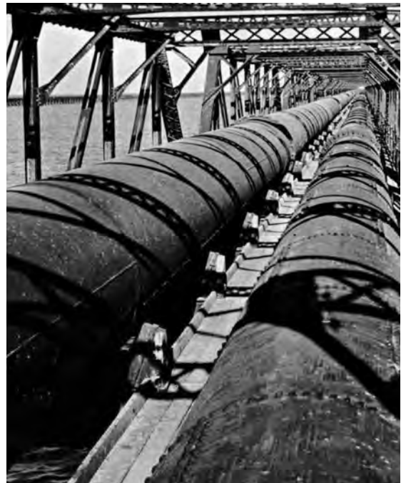
City of San Francisco, California – Bay crossing of the Hetch Hetchy Aqueduct. 66 inches diameter, 3/8-inch and 1/2-inch steel plate.
