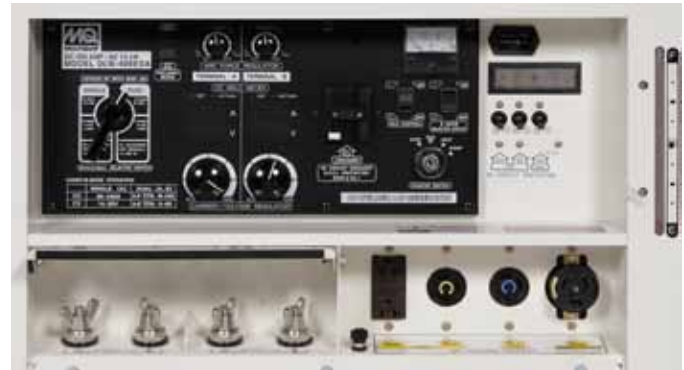
Full instrumentation is protected by a vandal proof cover. LED display provides clear readout of load characteristics.
