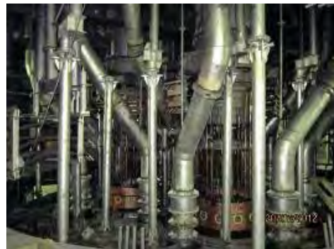
Calcium carbide furnace prior to commissioning.
