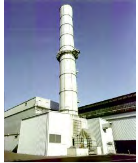
Gas cleaning plant.
