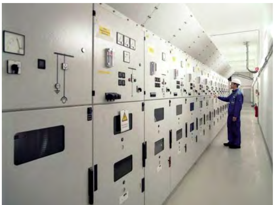
Power distribution room.
