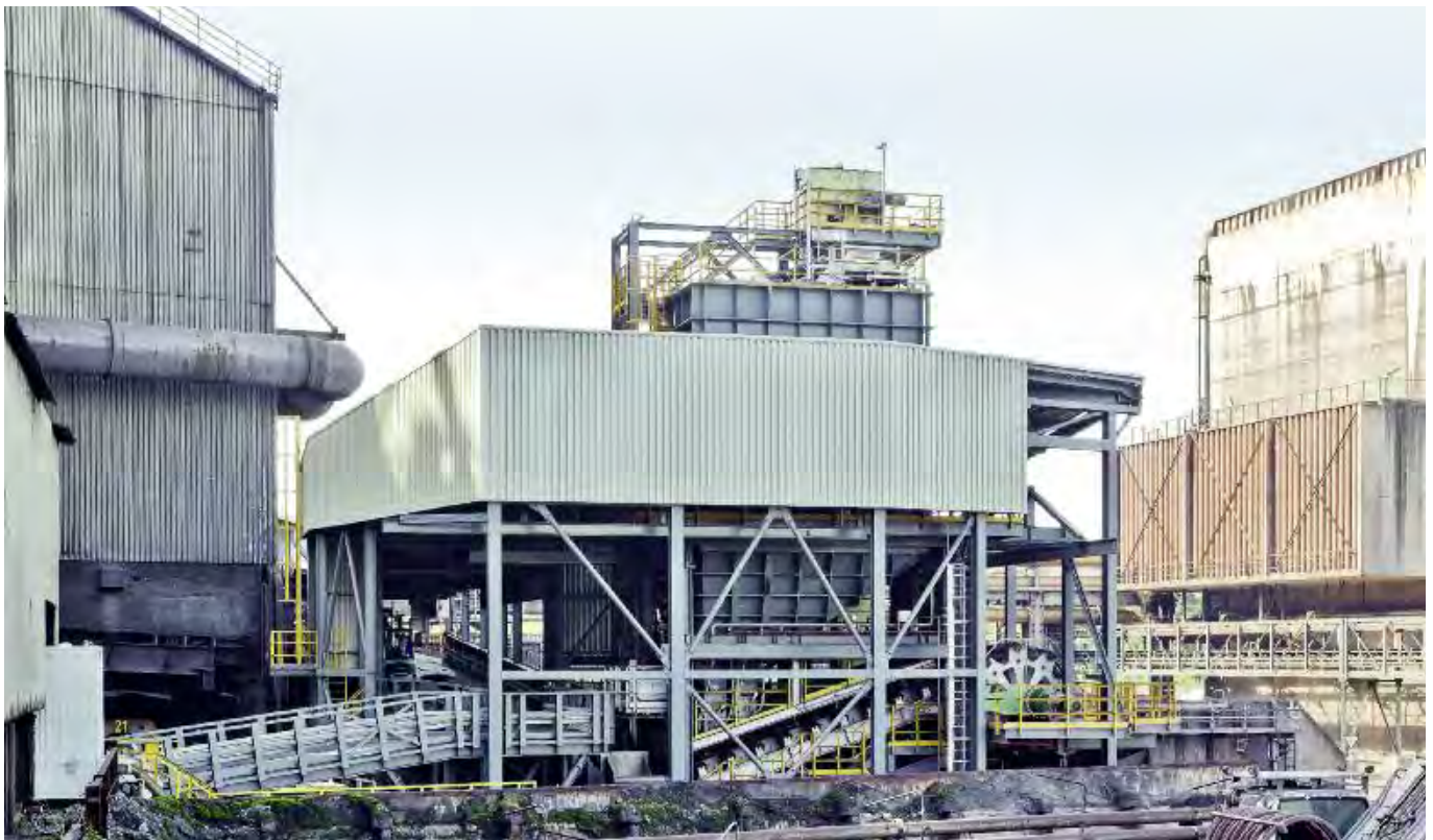
Dry slag granulation (Dillingen) Pilot plant.
