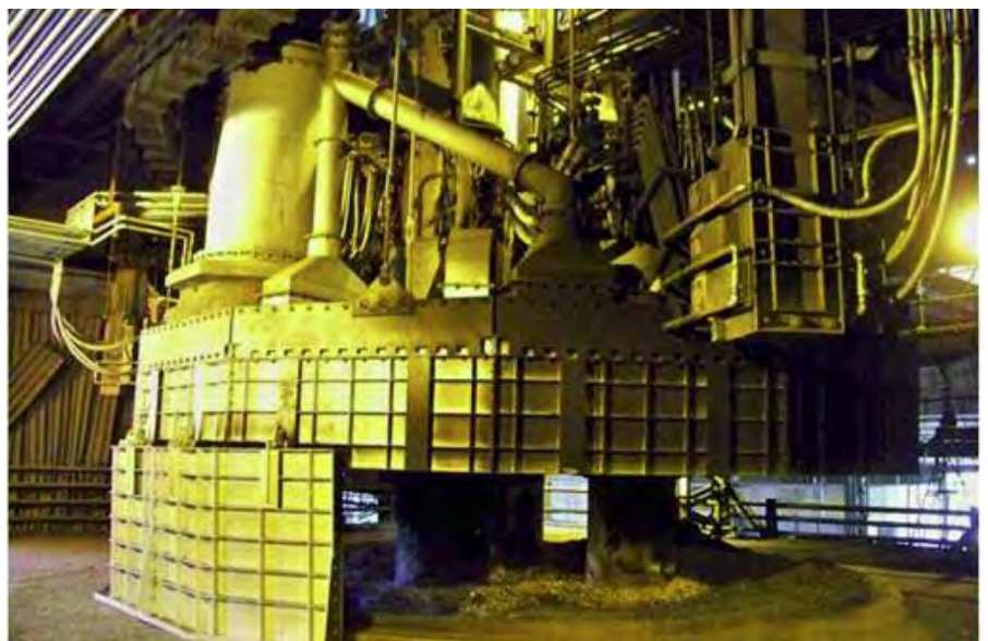
Mogale air cooled roof.
