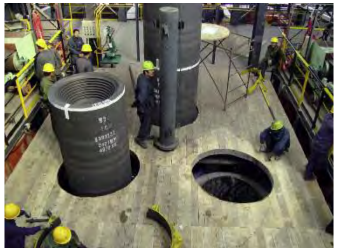
Nippeling area of a silicon furnace.
