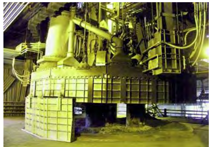
Air-cooled furnace roof.
