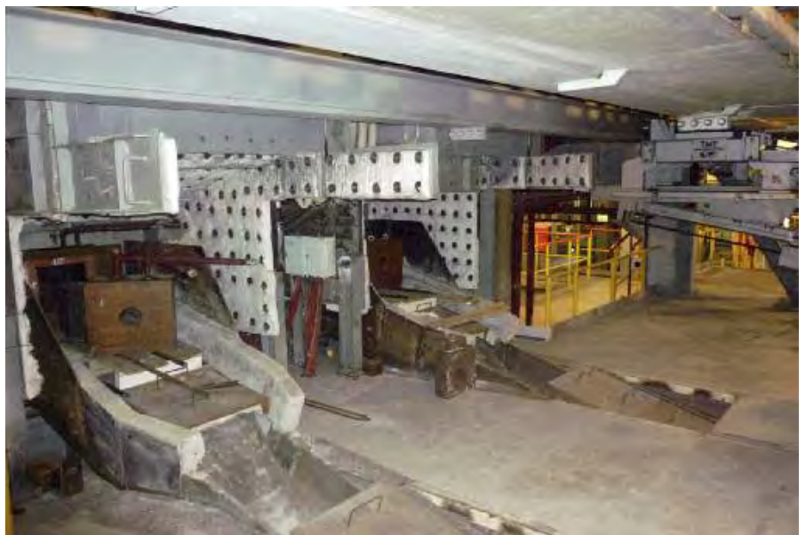
Tapping area of Kazzinc prior to commissioning.
