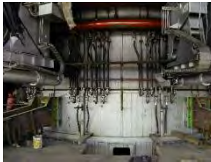
DC furnace for ilmenite smelting.
