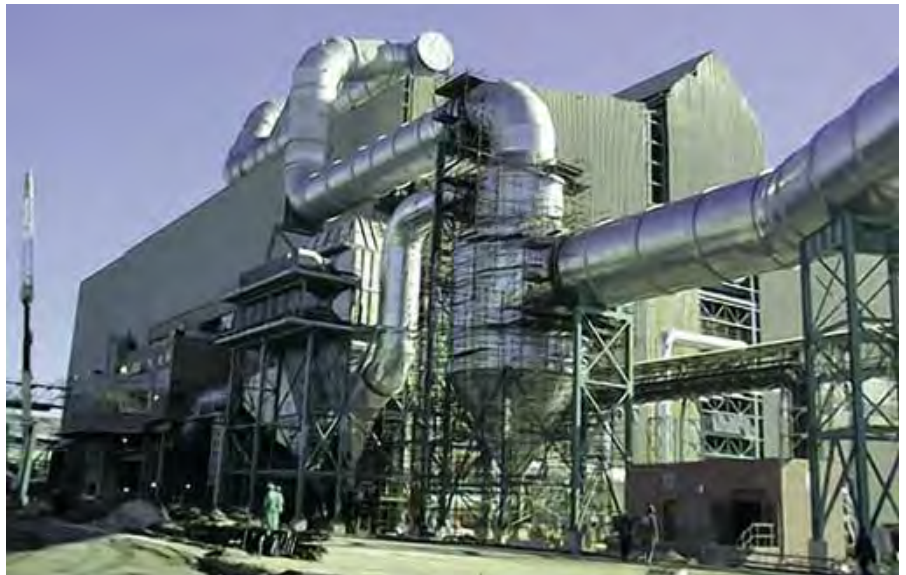
Gas cleaning plant.
