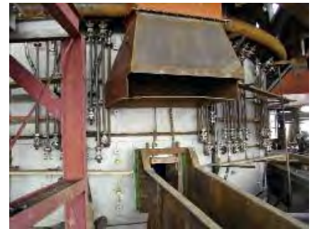
DC furnace for ilmenite smelting.
