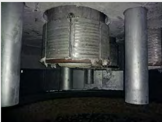
FeCr furnace at Etikrom prior to start up.
