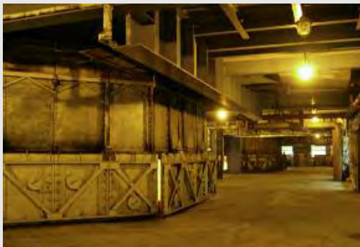
Furnace with doors for off-gas temperature control.
