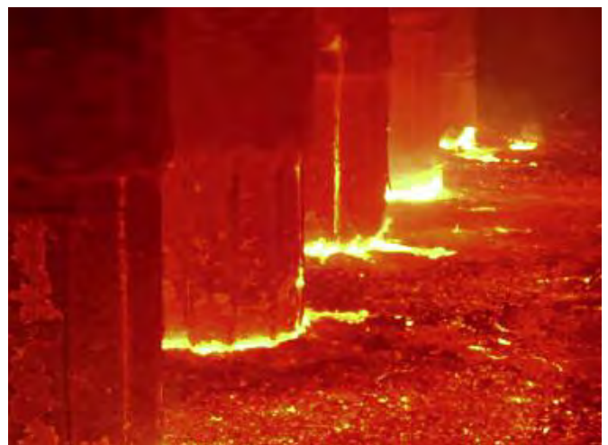
FeNi furnace inside view.
