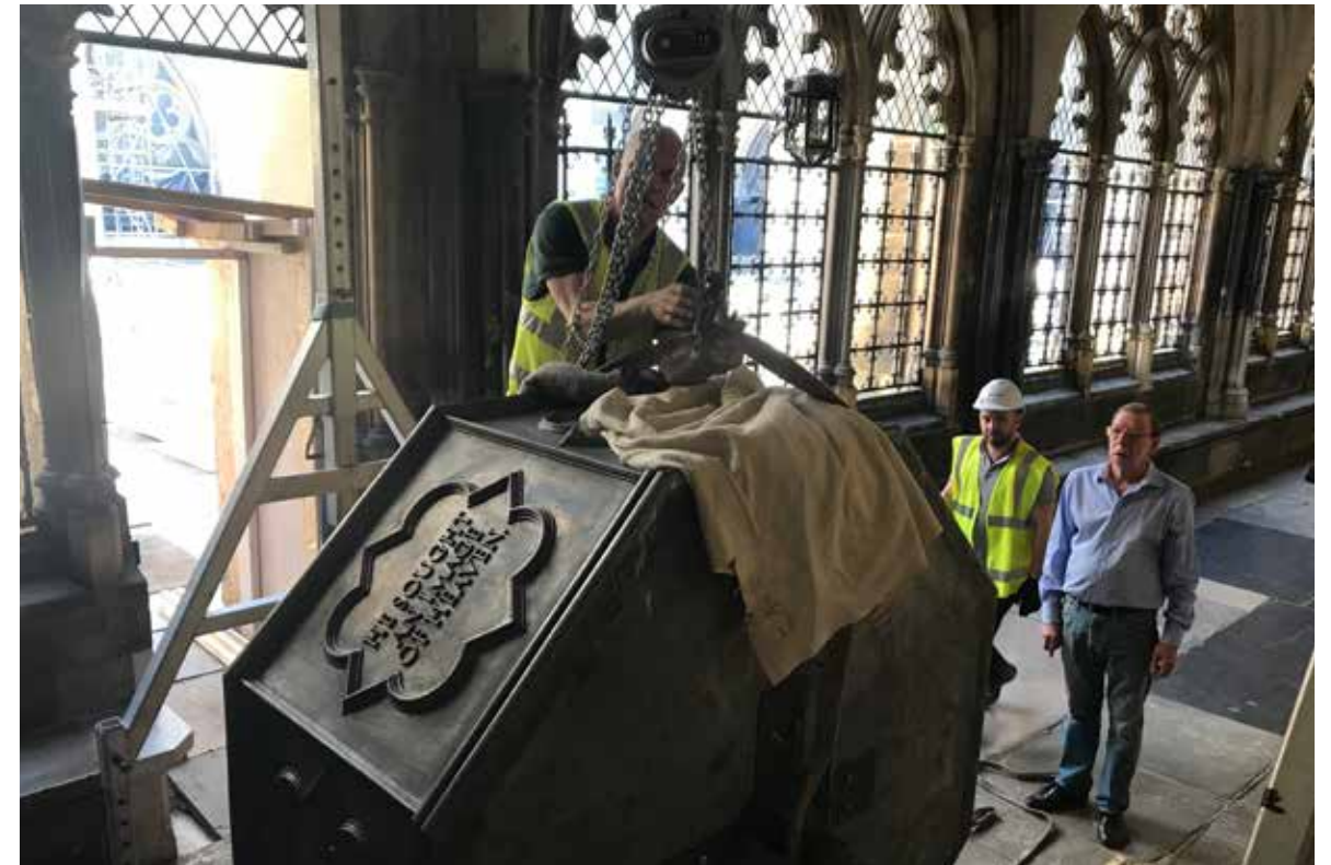
The Abbey's Clerk of the Works, Jim Vincent, supervises the installation of the new fountain installed in the Cloister Garth as a memorial to the landscape gardener Lancelot 'Capability' Brown.
