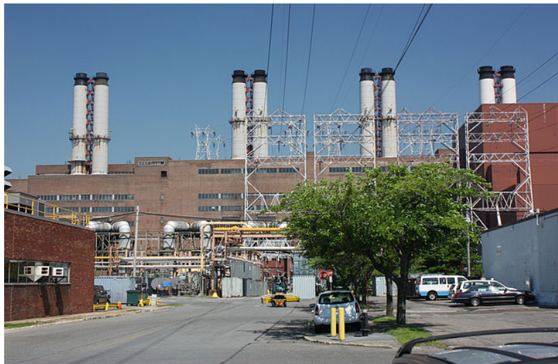
Modern microgrids can incorporate diverse energy sources, including natural gas as well as renewables.
