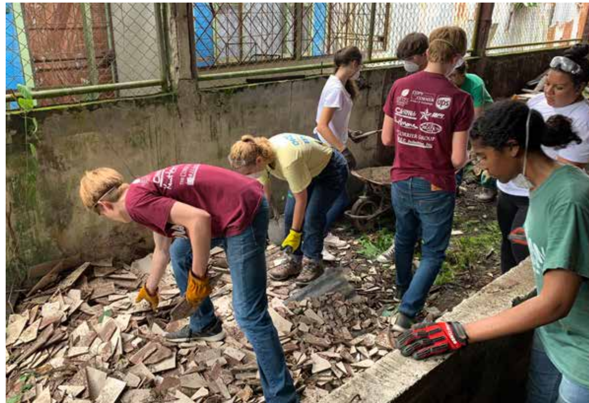
Below right: Cathedral youth in Costa Rica remove debris from the demolition of a church kitchen, with plans to rebuild a diocesan center nearby.
