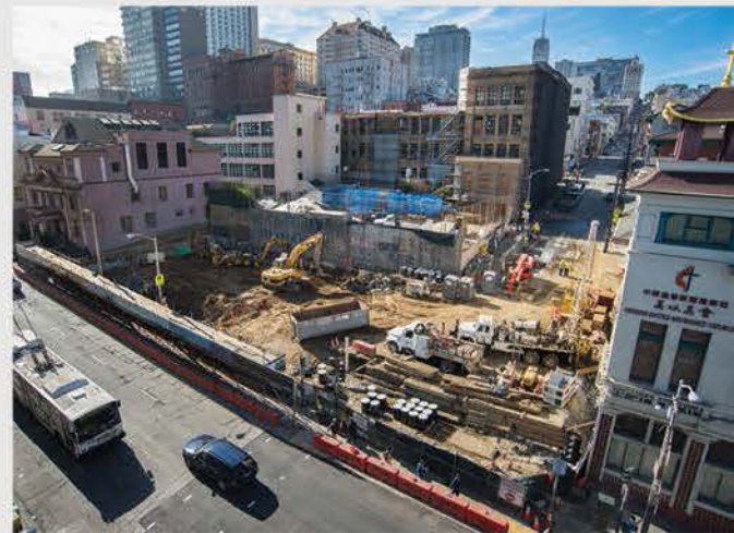
Central Subway station construction is underway in San Francisco Chinatown. (Photo: Courtesy of SFMTA)
