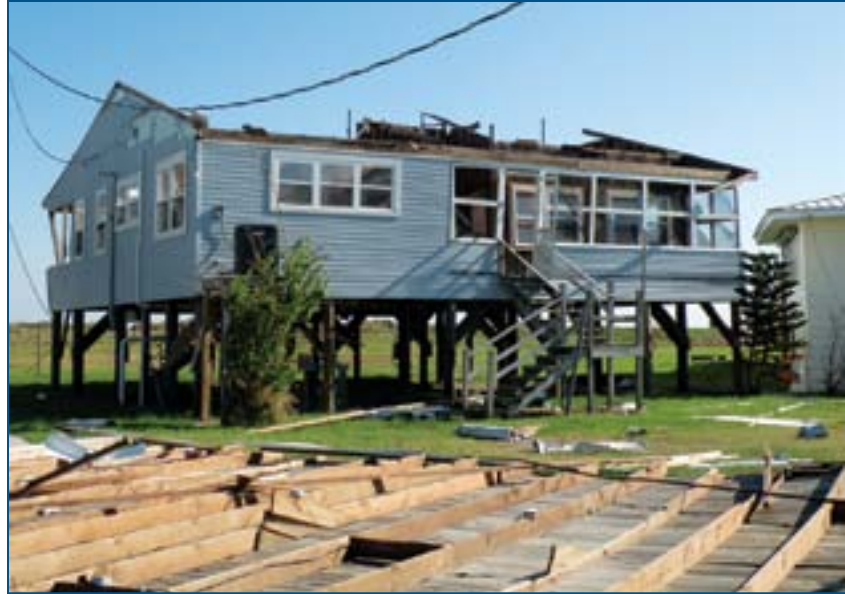
FIGURE 4-17: Roof structure that was poorly connected to the house (Jefferson Parish, LA) (SOURCE: FEMA P-757)
