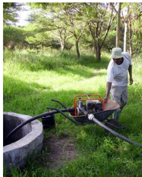
Figure 16. Diesel pump at ATC.
