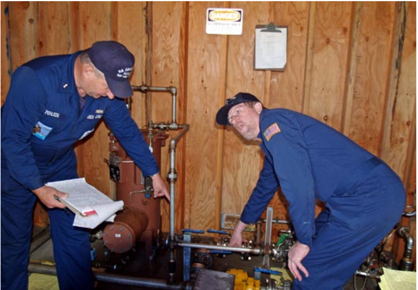
Doug Pohlson (left), FC-87, and Ken Reynoldson, FSO-CM 87 D11NR, identify the key valves in the fuel recirculation system.
