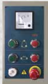
Conveyor speed control
