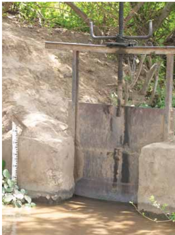
Figure 58. Some of the gates have measuring gauges even though they are not used at present.
