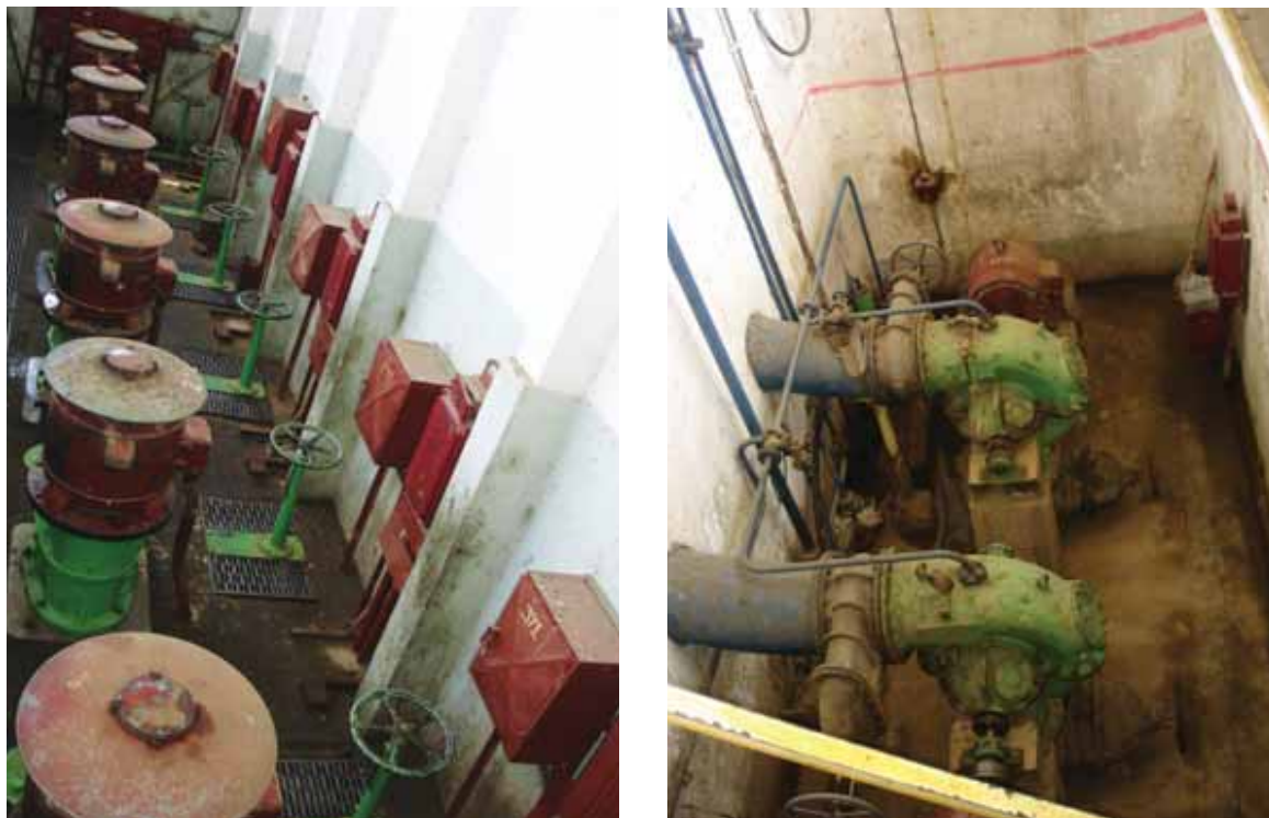
Figure 9. The main pump station at Wonji has eight pumps with design discharge of 55,000 liters per second (l/sec).
