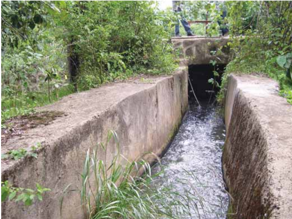
Figure 48. Rectangular main canal is used to convey irrigation water from the diversion.
