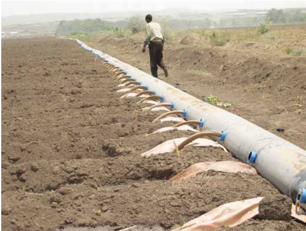
Figure 18. Recently, hydroflume has been introduced to replace feeder canals and siphons.
