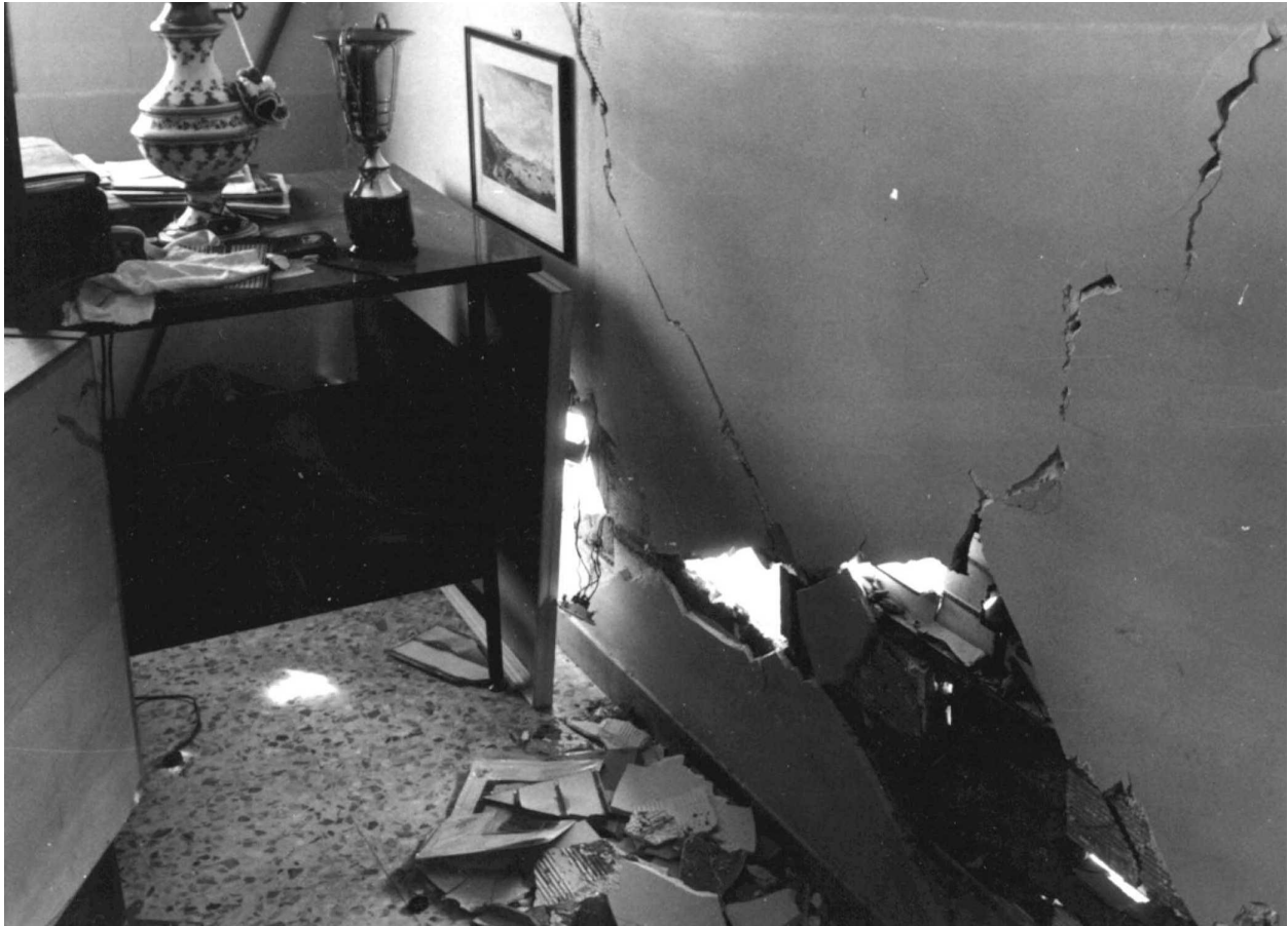
FIGURE 4B: Typical Earthquake Damage-Cracking of Masonry Partitions
