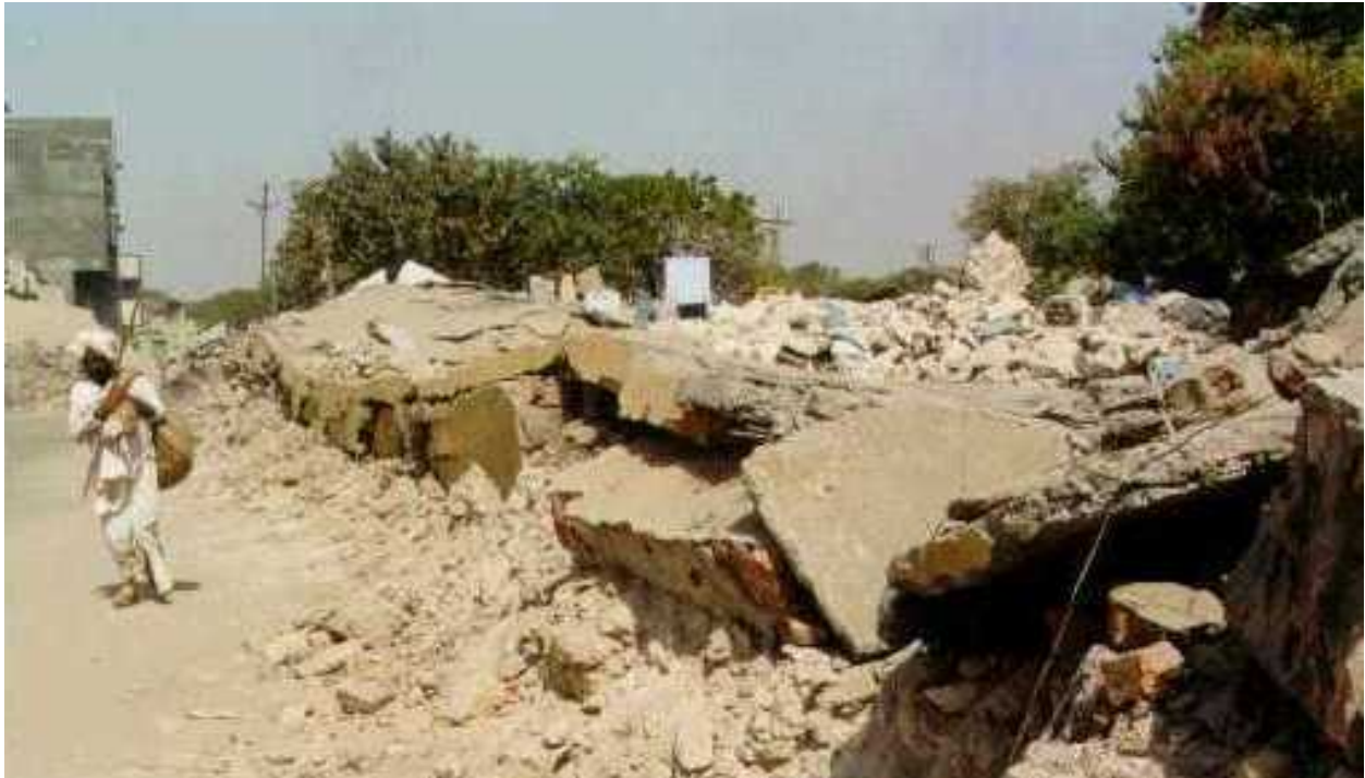
FIGURE 6I: Collapse of Brick Masonry Buildings in the 2001 Bhuj earthquake (Source: IIT Powai, 2001)
