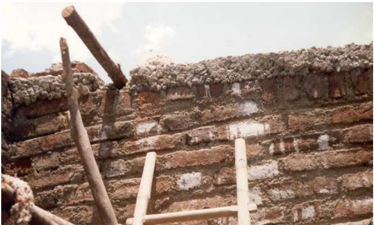
FIGURE 5C: Construction Deficiency - Discontinuous RC Lintel Band (bond beam)
