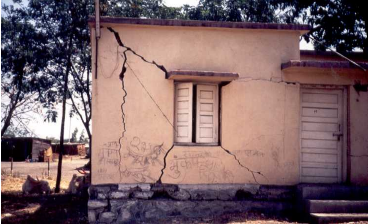
FIGURE 6F: Typical Earthquake Damage - In-Plane Wall Cracking(1993 Killari earthquake)
