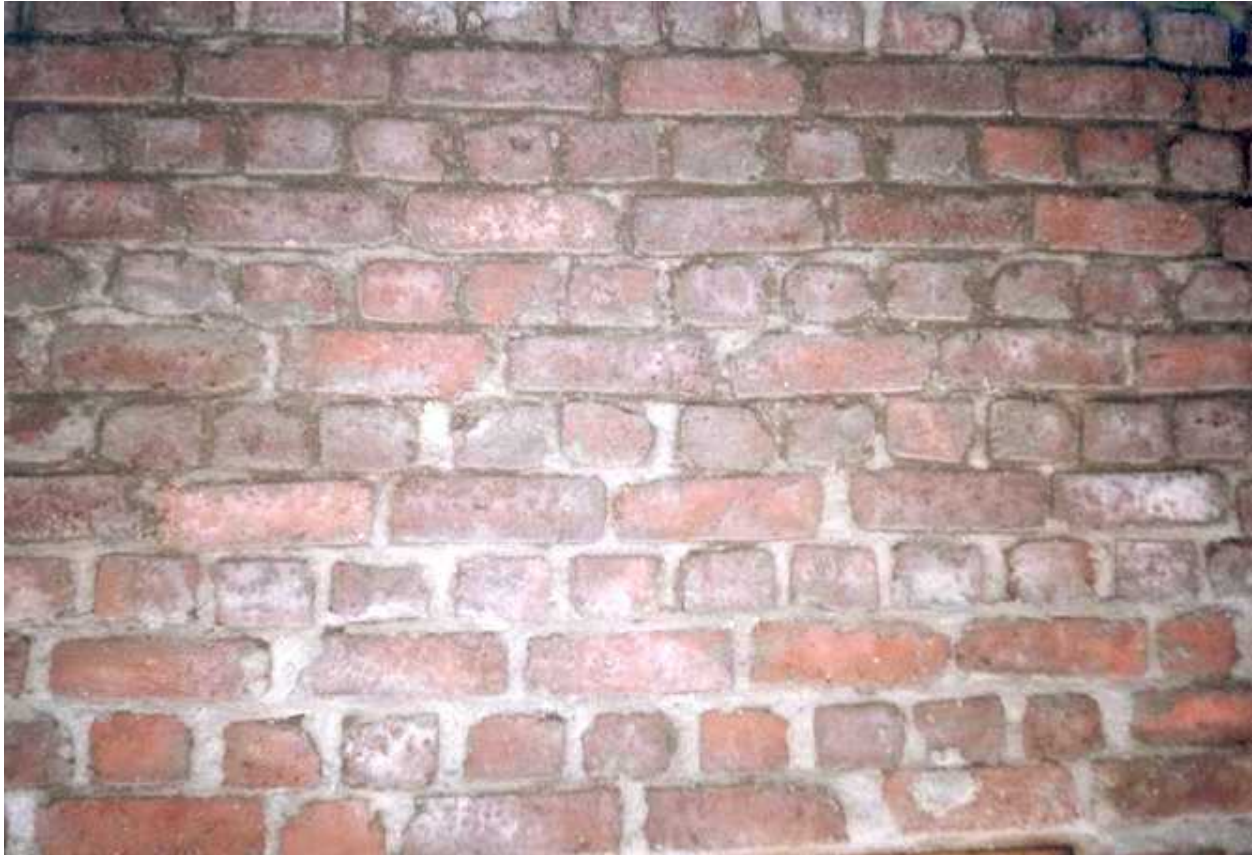
FIGURE 5B: Construction Deficiency - Excessively Thick Mortar Bedding Joints
