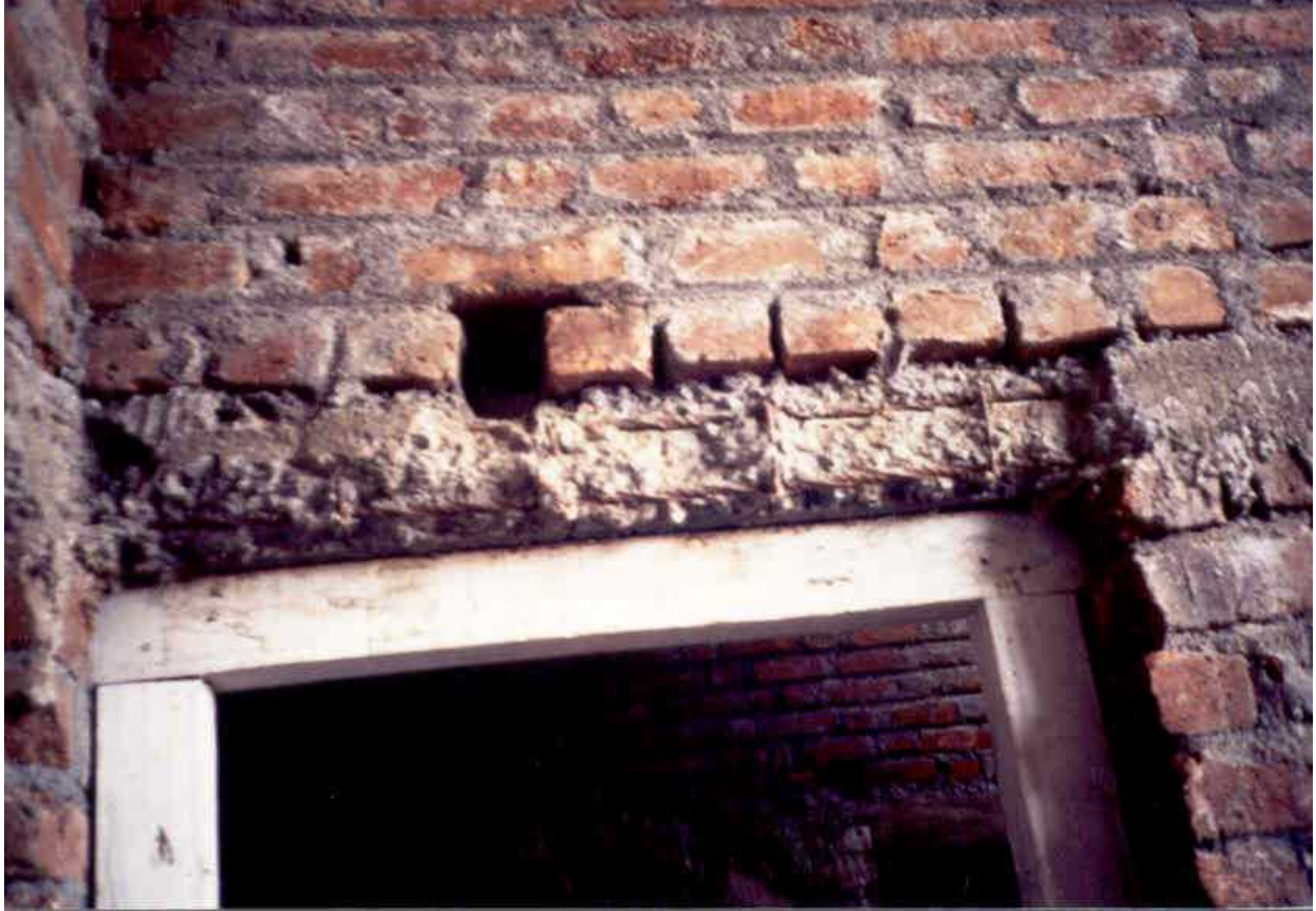
FIGURE 5E: Construction Deficiency - Exposed Steel Reinforcement in RC Lintel Band Construction
