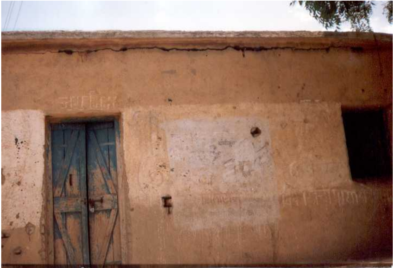
FIGURE 6E: Typical Earthquake Damage - Sliding Failure of Roof-Wall Connection Due to the Absence of Wall Reinforcement(1993 Killari earthquake)
