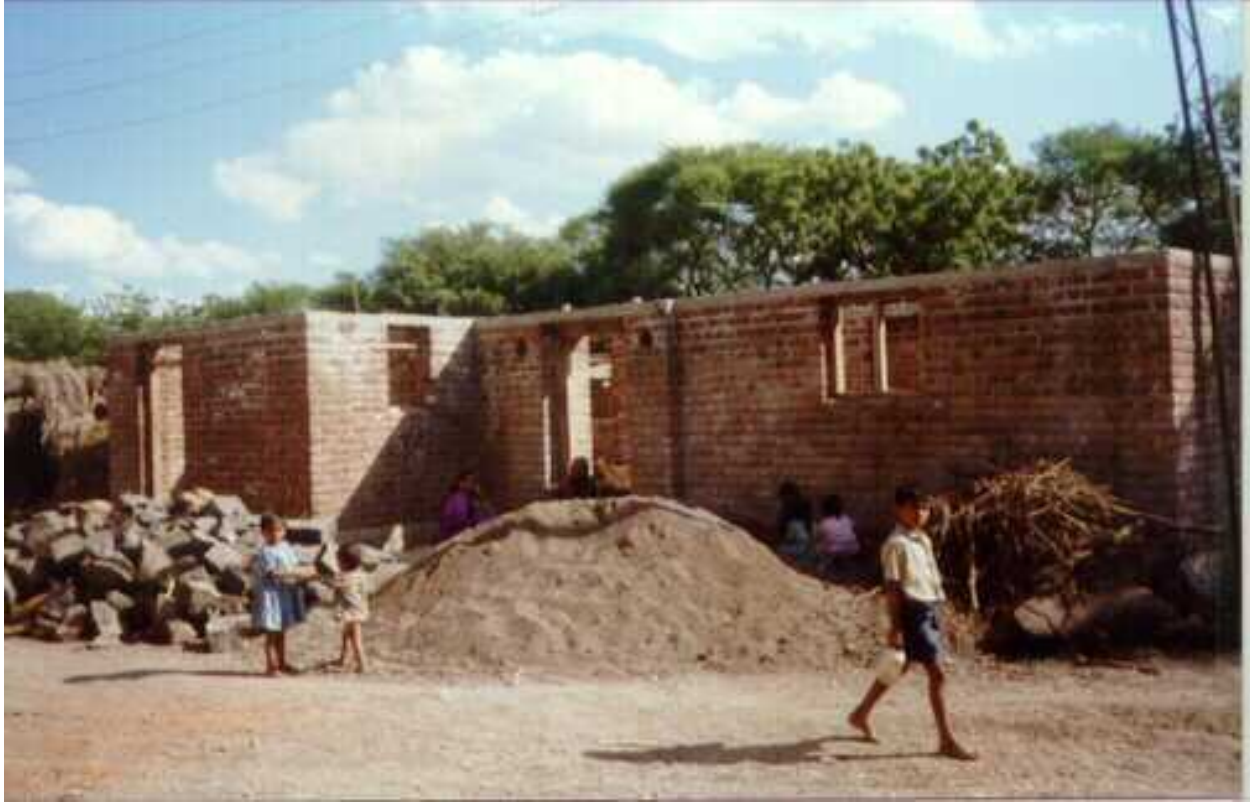
FIGURE 7D: An Example of New Construction with Seismic Features (note RC lintel band)
