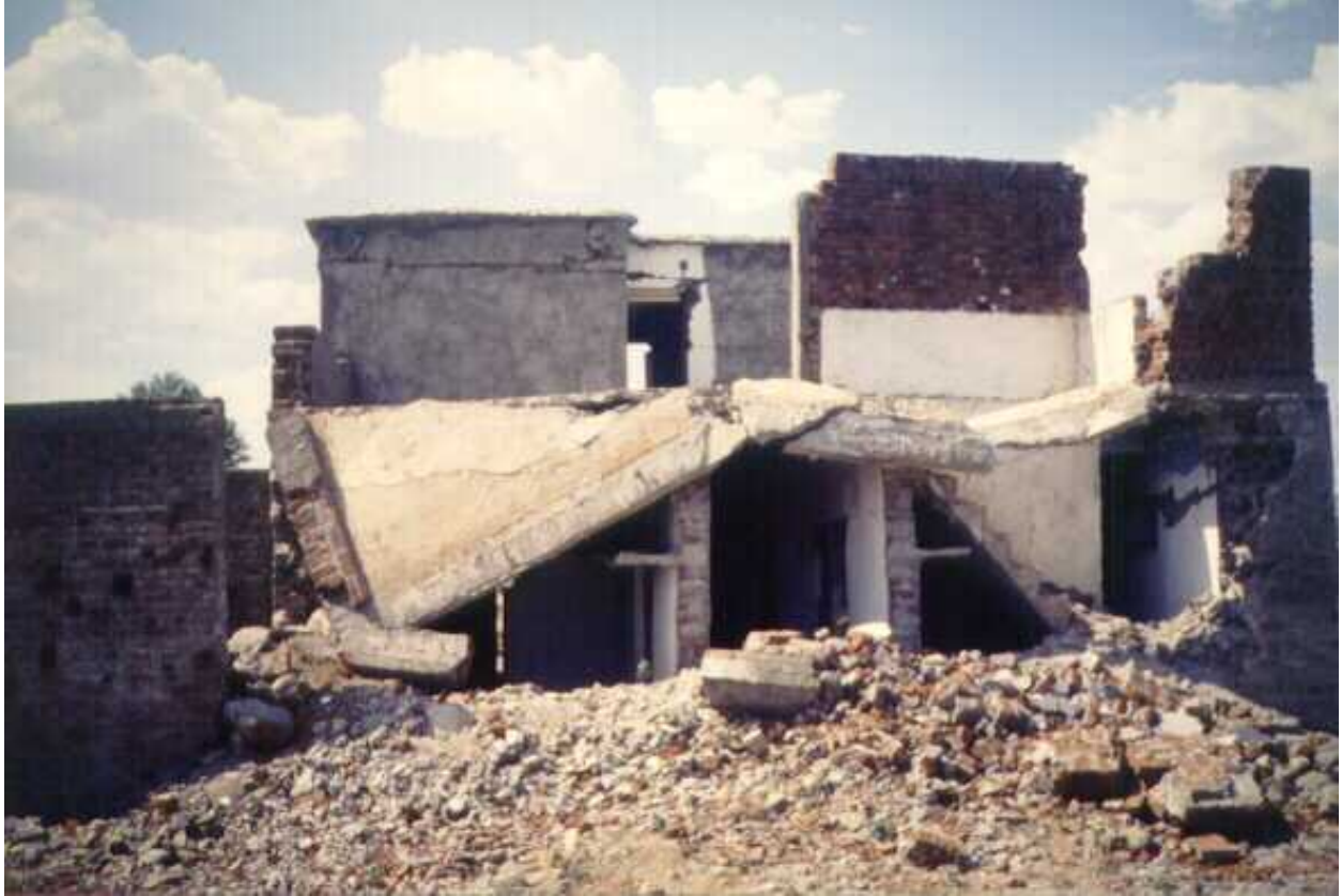
FIGURE 6a: Typical Earthquake Damage - Roof Collapse Caused by the Wall Collapse (1993 Killari earthquake)
