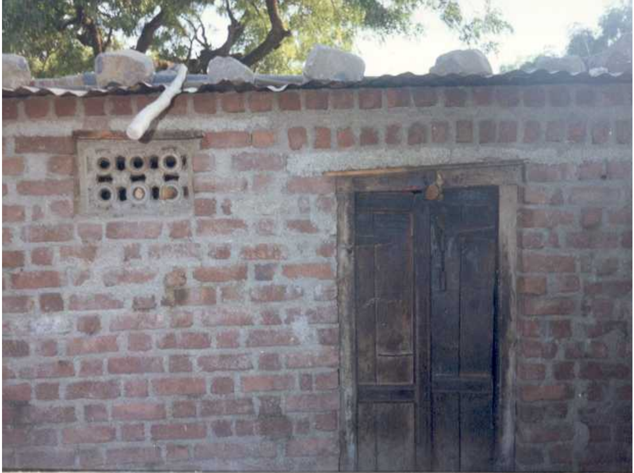
FIGURE 5D: Construction Deficiency - Discontinuous RC Lintel Band
