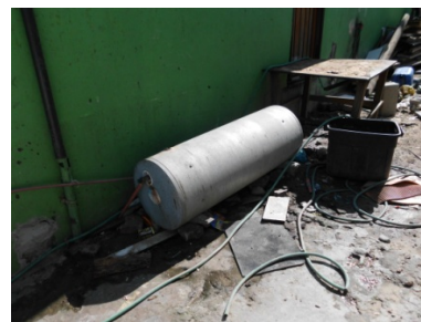
A typical hot water installation ☹
