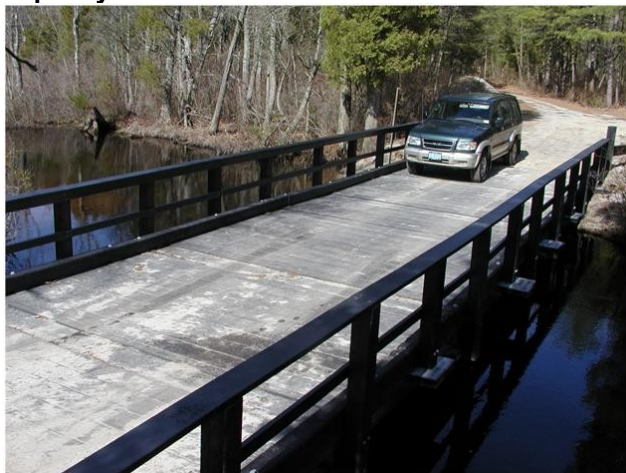
Figure 2. Vehicular bridge in Wharton State Forest, New Jersey built in 2002 with an I-beam substructure and a maximum load capacity of 36 tons.
