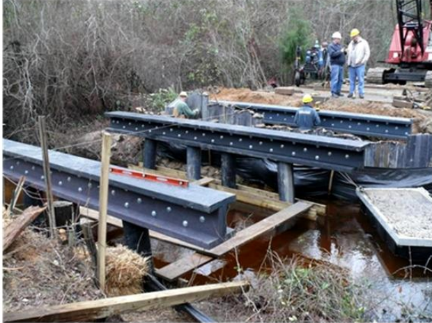
Figure 7. Pile caps in place and pinned on three rows of pilings on T85-18.
