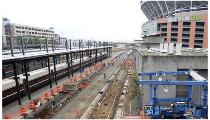
Work continues on the King Street Station track upgrades in Seattle; the project is expected to be completed in spring 2017.
