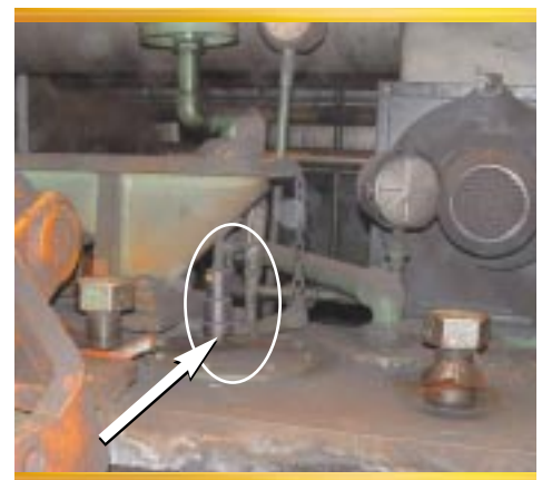
Hydrolert Transducer installed on a bank of rollers at a steel mill facility.
