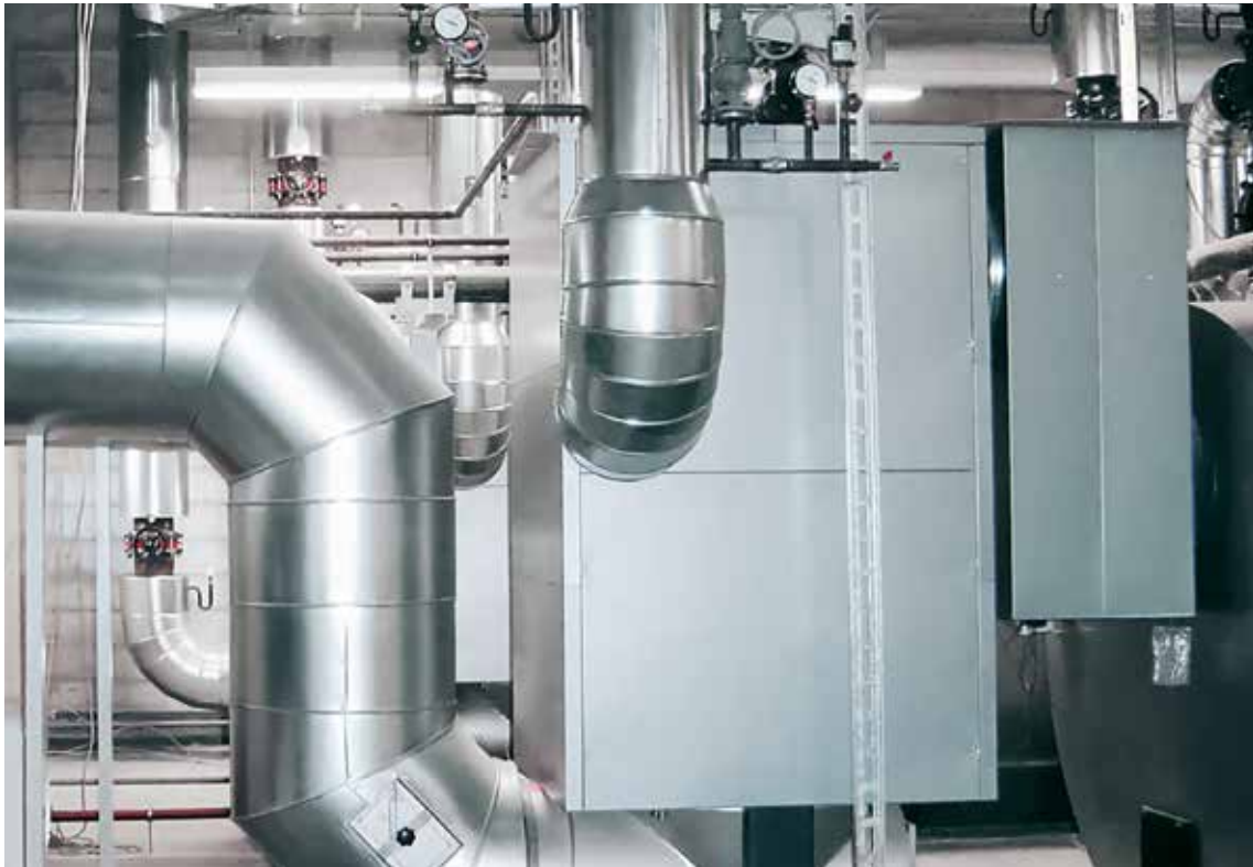
Downstream Vitotrans 300 heat exchanger fitted to a Vitomax boiler
