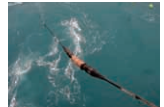
Submarine cable system
