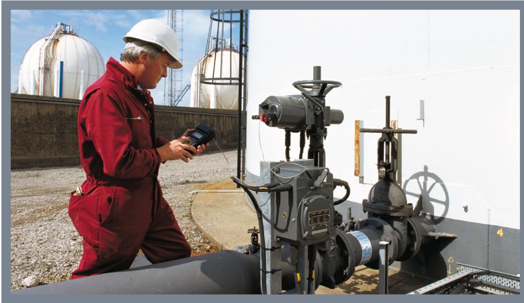
John Pratt performs the 'non-intrusive' commissioning of an IQ Mk 1 actuator inside the hazardous environment of an oil storage depot
