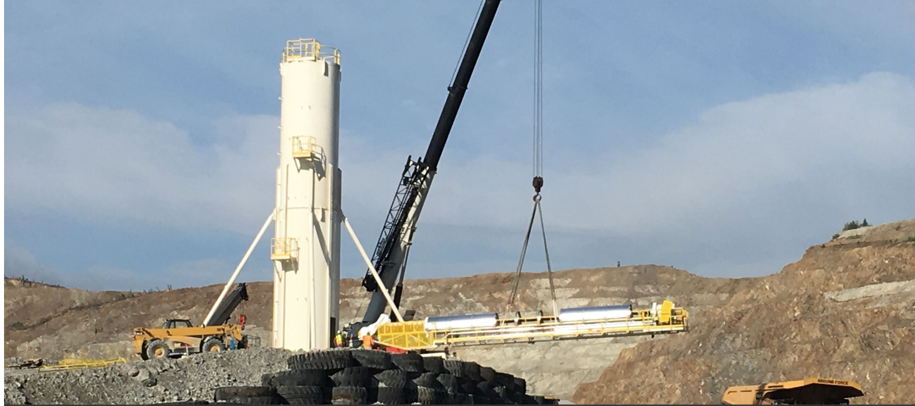
Manufactured Lime Silo and Discharge Conveyor
