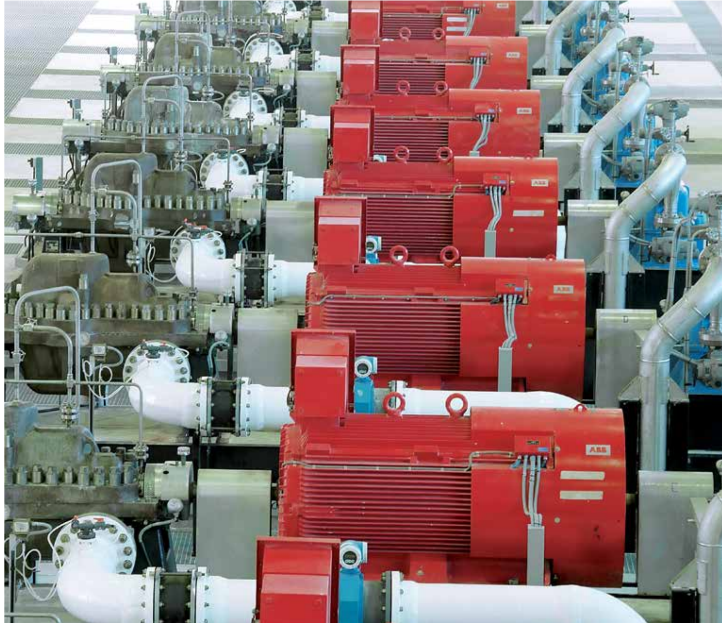
Desalination plant in Alicante, Spain
