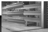
Stay within the yellow lines, use the small doors and do not touch components
