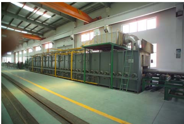
Natural Gas Stabilization Heat Treatment Furnace
